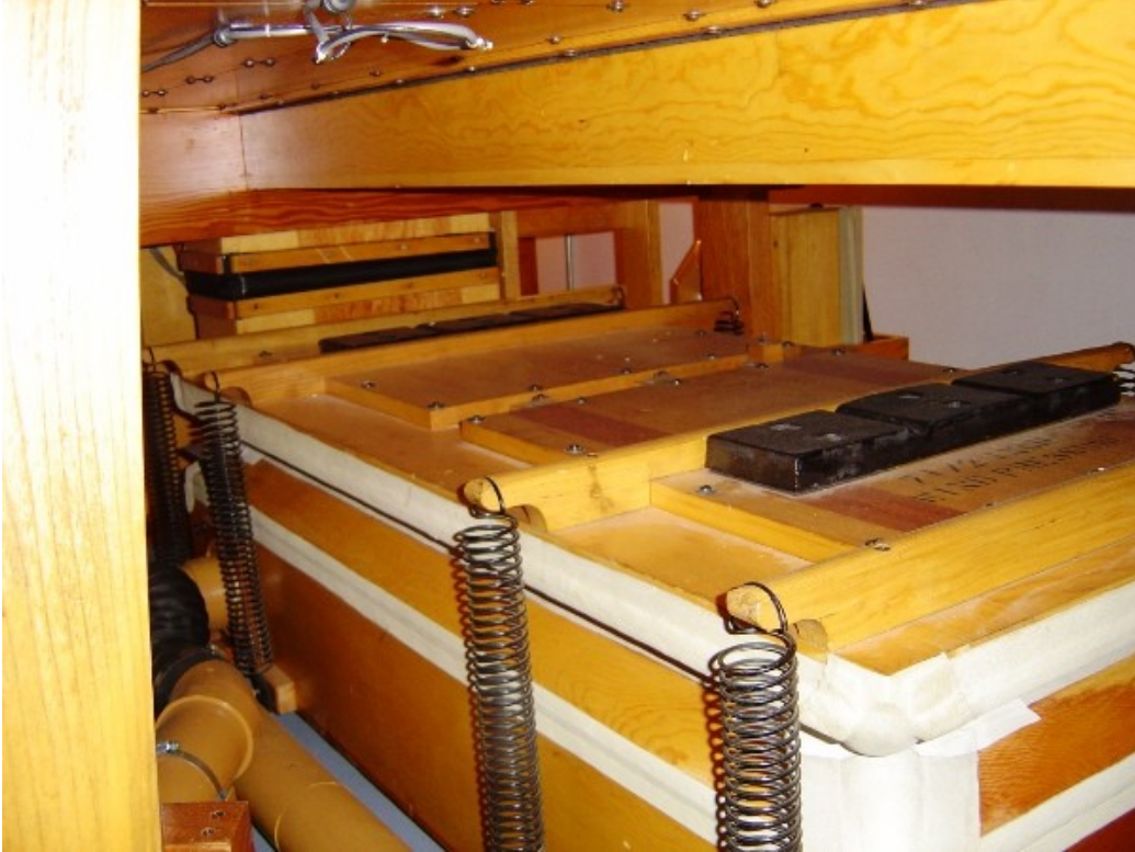
Figure 5: Reservoirs on the floor under the lower Swell windchest
