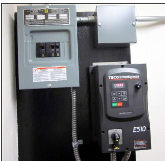
New, modern electrical circuits, replacing fuses from the 1950's. The VFD is shown at right.
